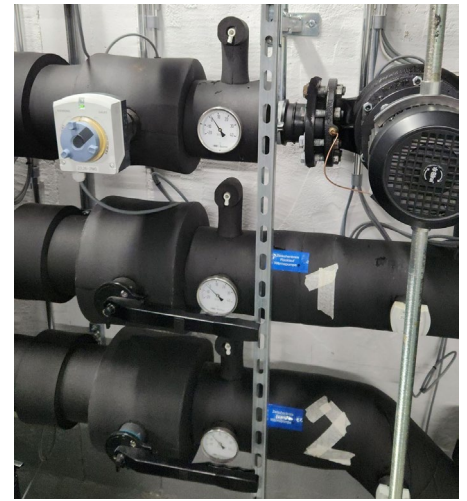
Supply and return lines of heat pumps 1 and 2.
