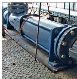
Pumping substrate between fermenters
