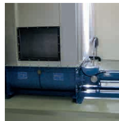
Conveyance of dewatered sewage sludge from decanter for drying: KL65R80.2 Triplex progressing cavity pump
