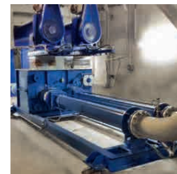
Conveyance of dewatered sewage sludge: KL80RQ110.4+110.4 Progressing cavity pump
